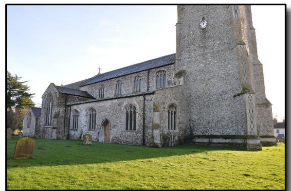
The north wall in its entirety and, in the open angle created by the junction of the tower's north wall and the west end of the north aisle, we find another conundrum as shown in the picture below.
